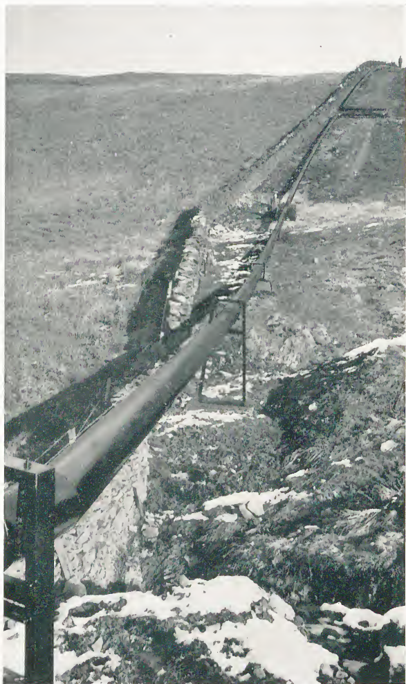
18 inch 'S & L' steel pipes with welded joints forming part of the South Wales gas grid.
